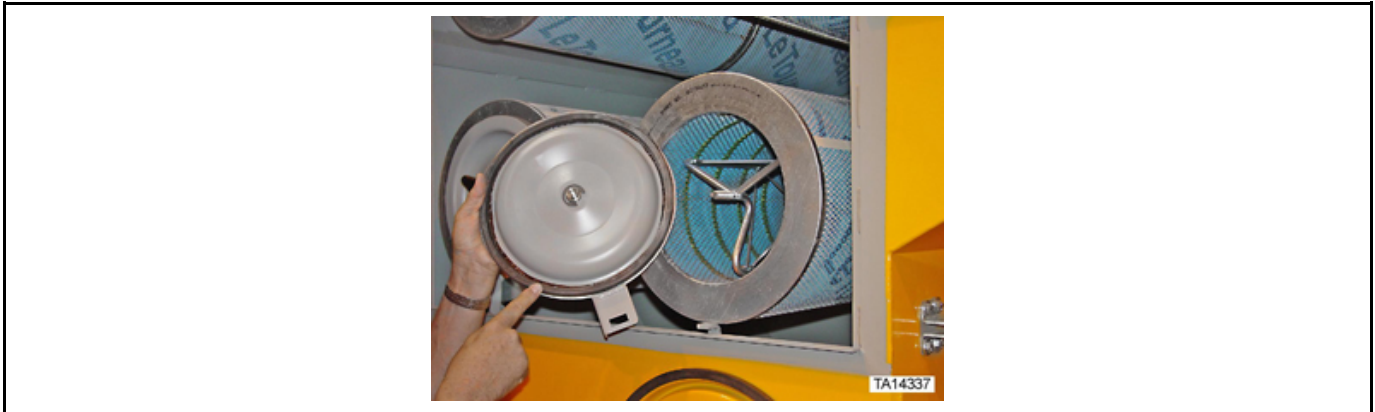
Figure 100: Inspection of tabbed cover gasket
