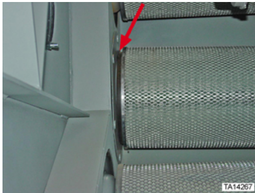
View through clean air chamber external door
